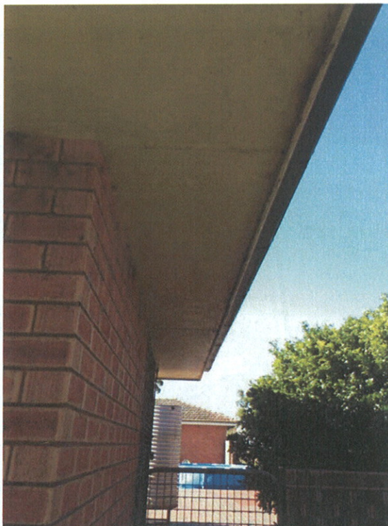
Photograph 25 – Suspected ACM eaves of the brick building on western corner of the complex, looking north.
