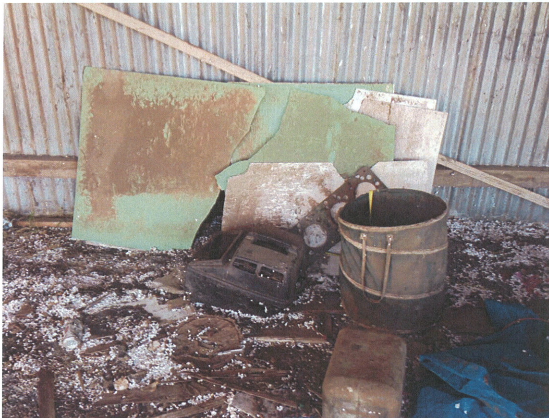
Photograph 50 – ACM inside the shed southwest of residence 3.
