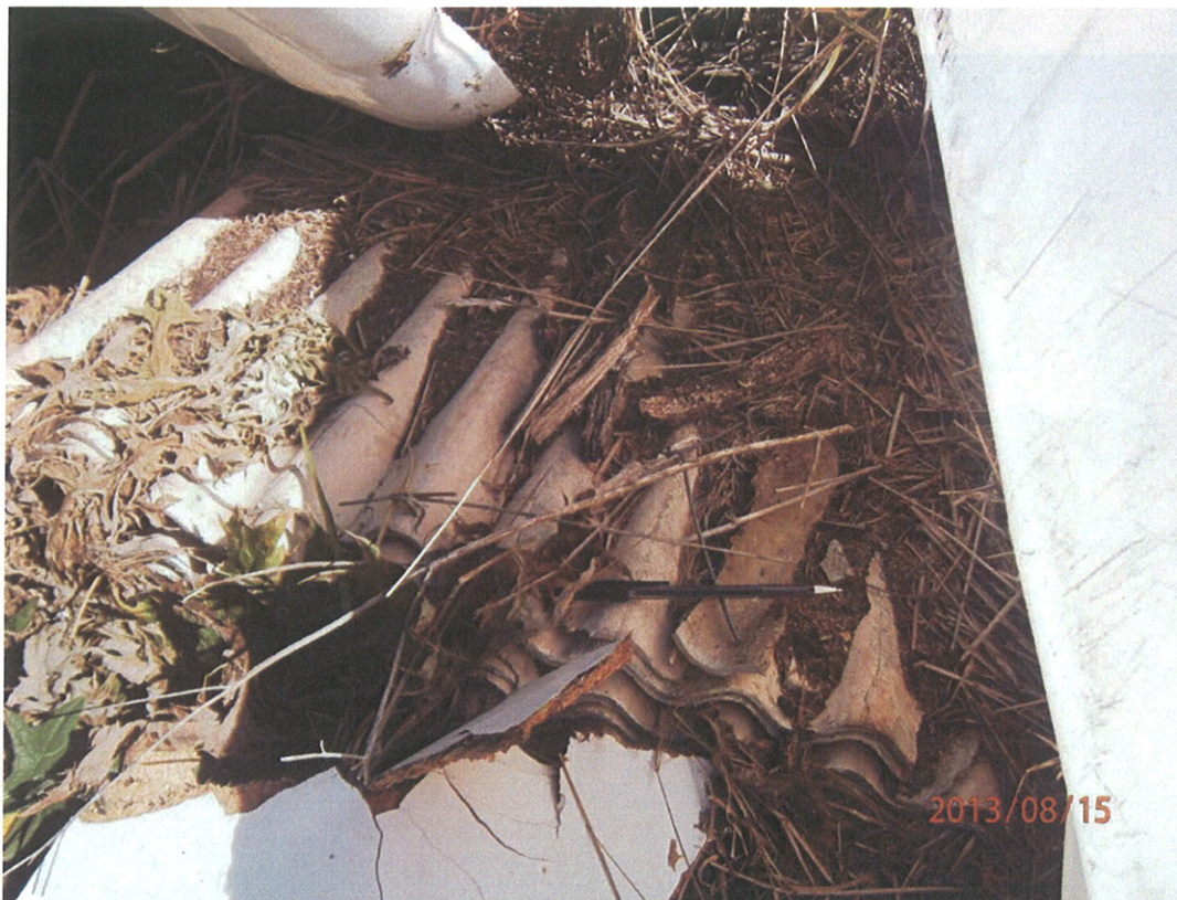
Photograph 19 – ACM sheeting stockpiled west of the house in the southeastern portion Lot 201
