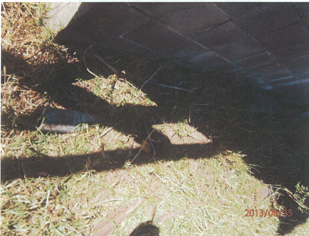
Photograph 16 – ACM drainage pipe at the rear of the Stable shed in the northeastern portion of Lot 201
